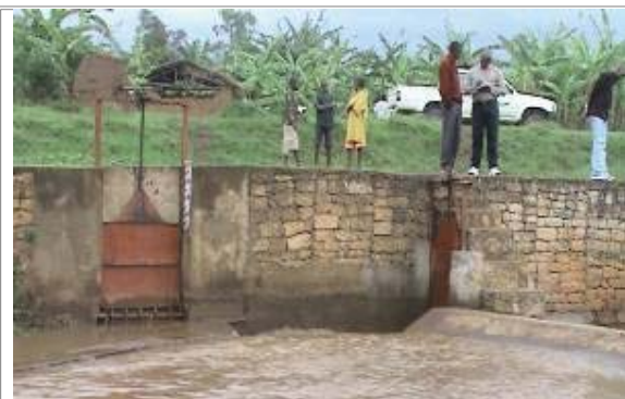
Figure 13 : Upstream view of the irrigation dam on the Muyogo river (Rukoziri area in MAKAMBA)
