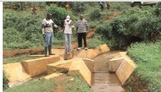
Figure 34 : Gates stolen on a small dam (Kadohaka river in KARUZI)
