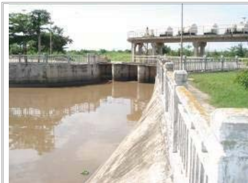
Figure 17 : General view of the diversion dam on the Mpanda river (RUKARAMU area)
