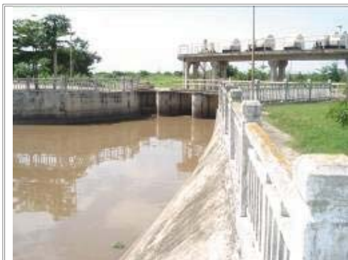
Figure 12 : Upstream view of the irrigation dam on the Mpanda river (RUKARAMU perimeter)
