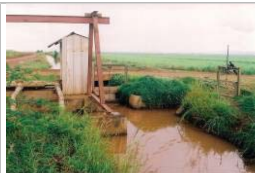
Figure 21 : View of the pumping station on the main canal (SUCOMO)
