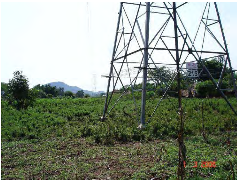
Photo 3. Existing transmission line coming out from Tororo substation
