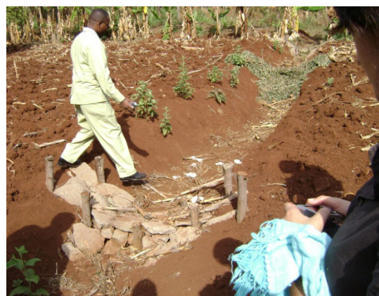
Figure 4.3 (a) Sketch of artificial waterway with drop structures made with logs (b) Drop structures made of local materials ( photo courtesy of Faith Muthoni )
