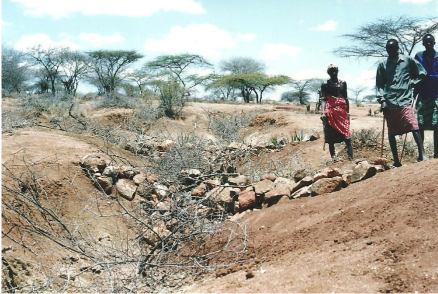
Figure 5.6 Gully control with stone check dams and brushwood fills (photo by B. Mati)
