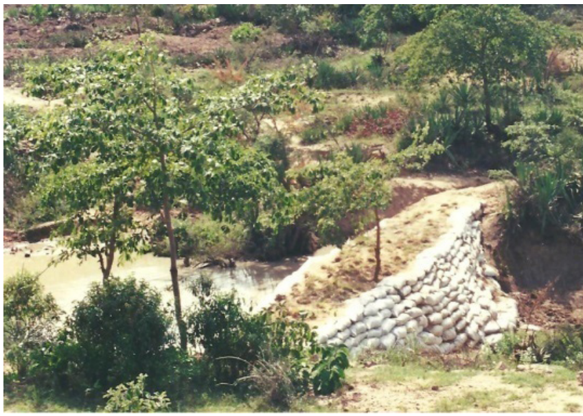
Figure 5.4 Gully control with cushion check dams (soil filled bags) (Photo by B. Mati)
