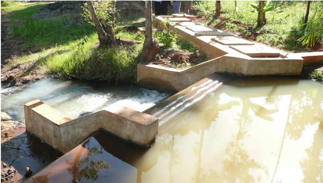
Figure 3.3 Broad-crested weir with stilling pool and diversion boxes (photo by B. Mati)
