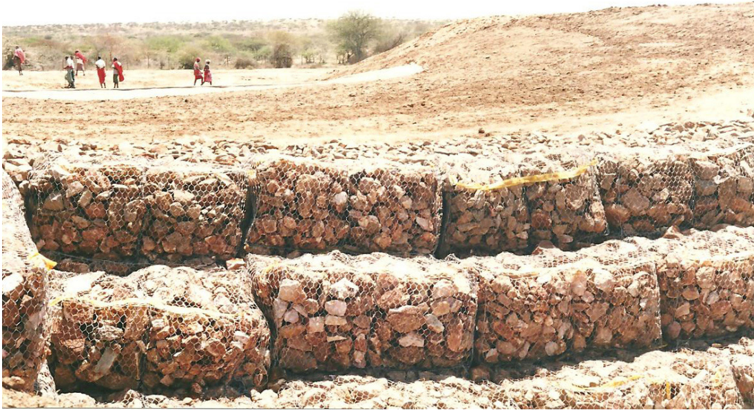
Figure 3.5 View of a gabion check dam across a dry valley (photo by B. Mati)
