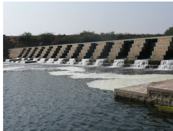
(b) Downstream side of same barrage with a set of self-cleaning spillways
