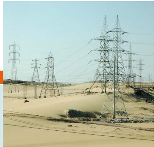
Electricity pylons, Egypt.
