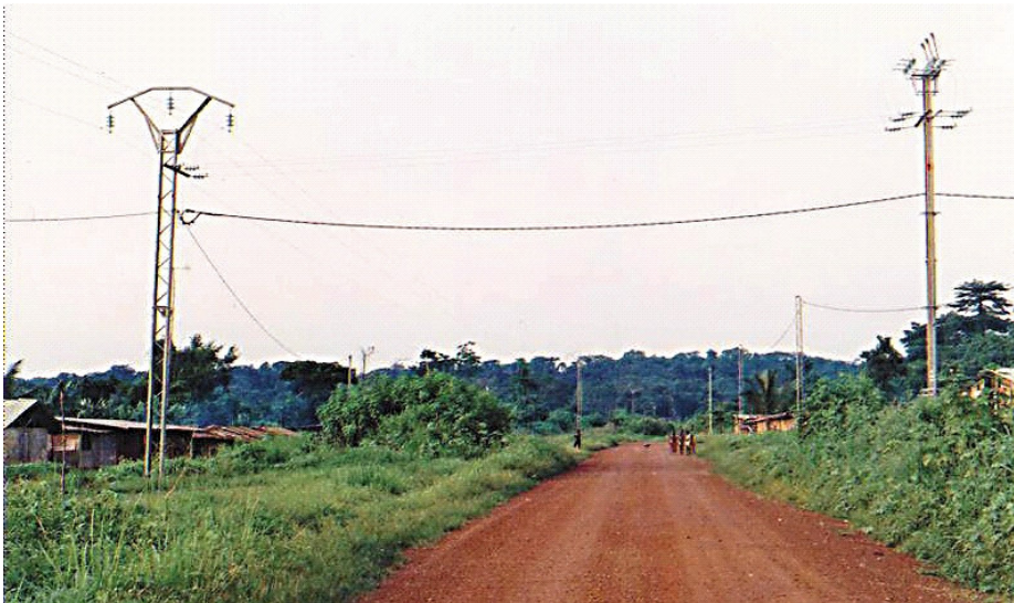
Power distribution line
