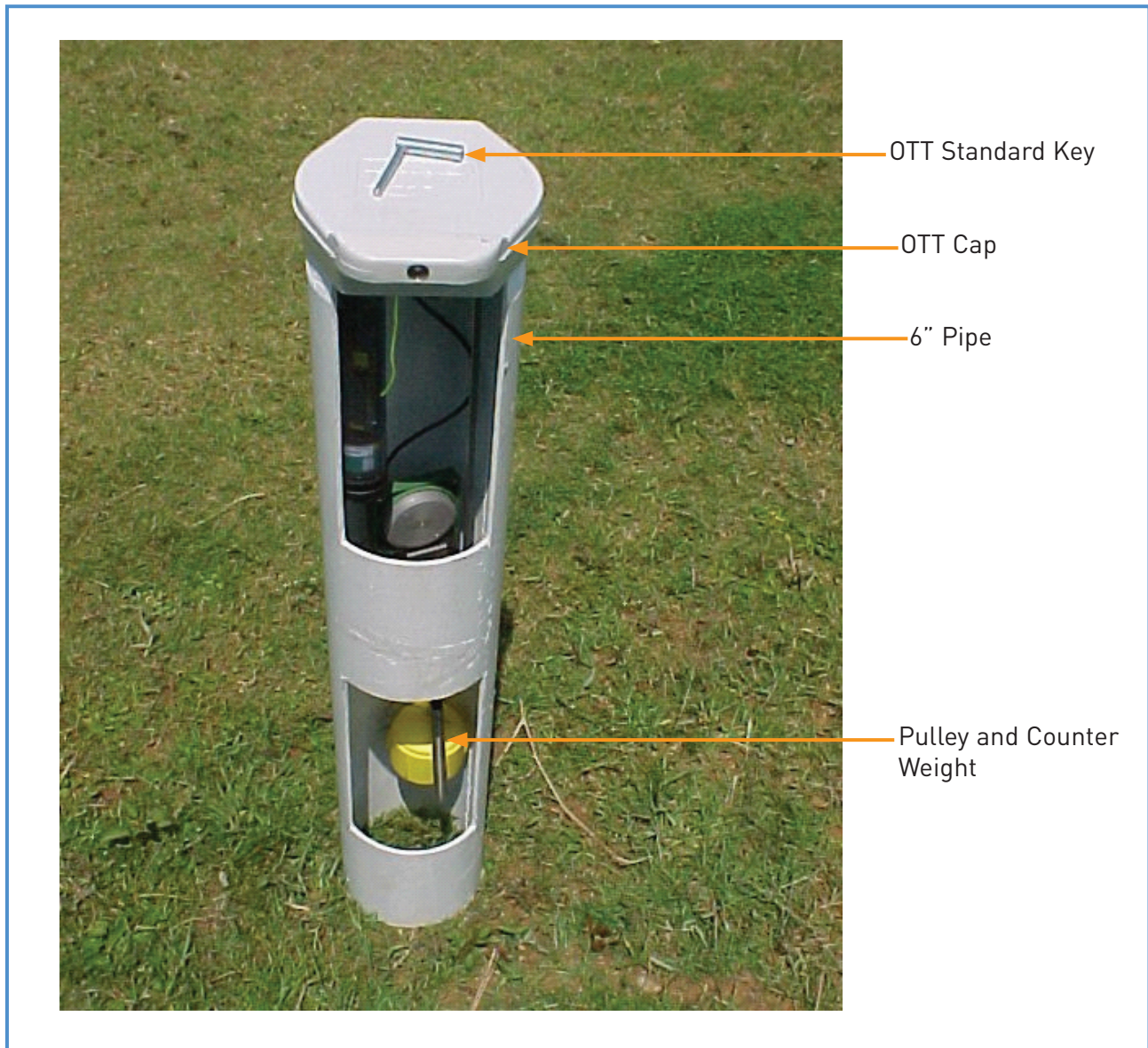
Figure 10: Thalimedes installed in a 6" demonstration pipe.
