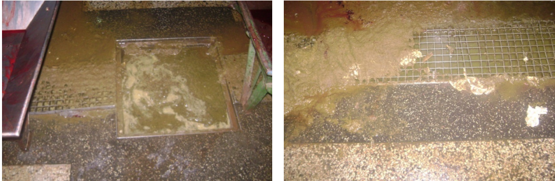
Figure 3.3: Wastewater from the evisceration process
