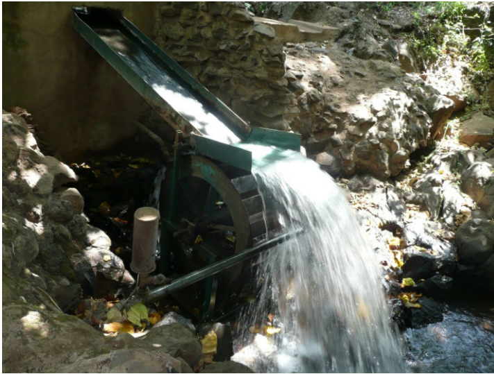
Figure 7.5 A hydram pump installation in a river (Photo by B. Mati)
