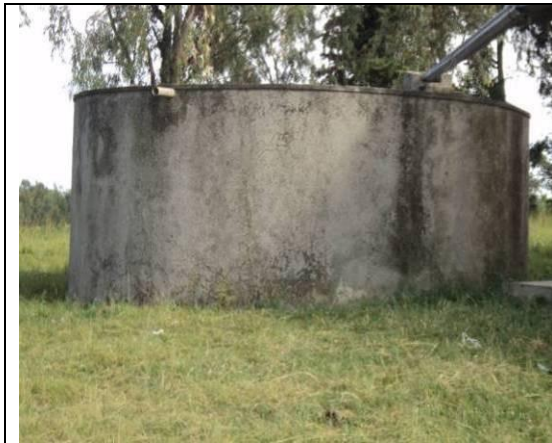
Plate 6-39: Water tank at Kashumba sub-county
