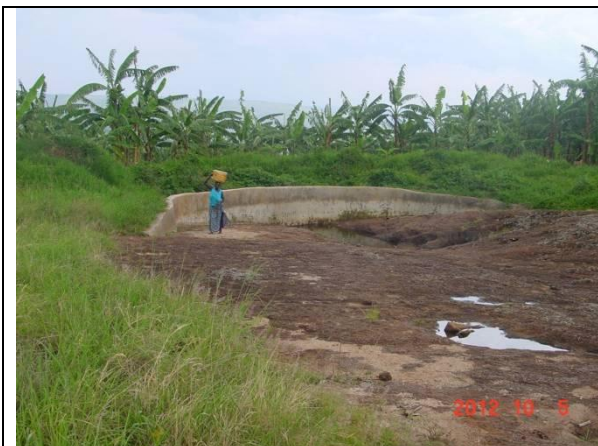
Plate 6-18: Rock water harvesting tank
