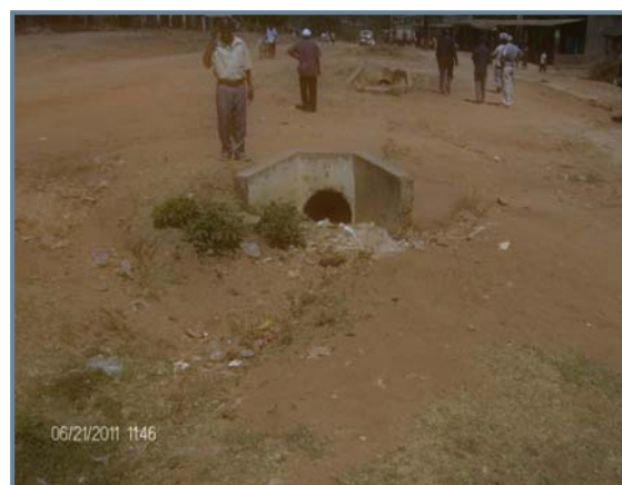
A poorly maintained access culvert on the Kenyan side
