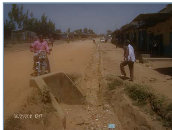
A section of the main drainage channel alongside the main road on Uganda side. Note well maintained cross culvert
