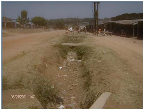
A section of the drainage channel along the main road on the Kenyan side
