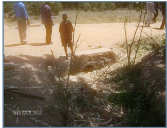
A poorly maintained undersized cross culvert on the Ugandan side.
