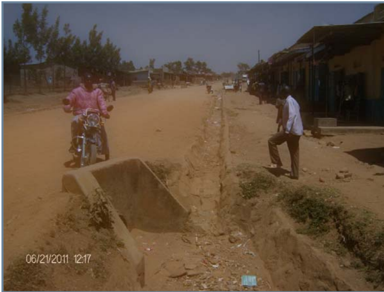
A fairly well maintained lined channel and cross culvert on the Ugandan side
