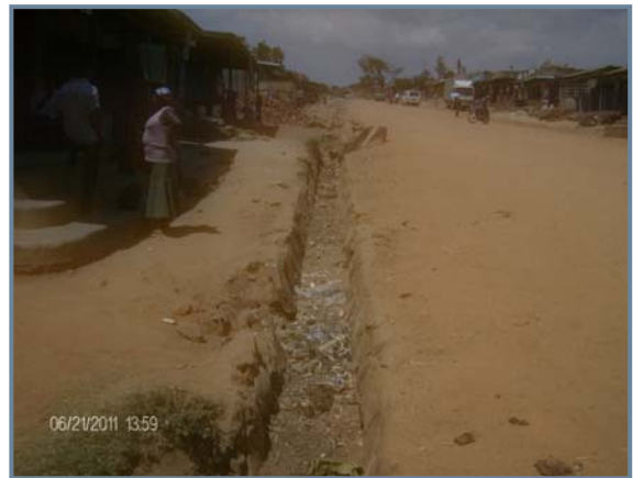
Stone pitched open drainage channel on the Uganda side of the town
