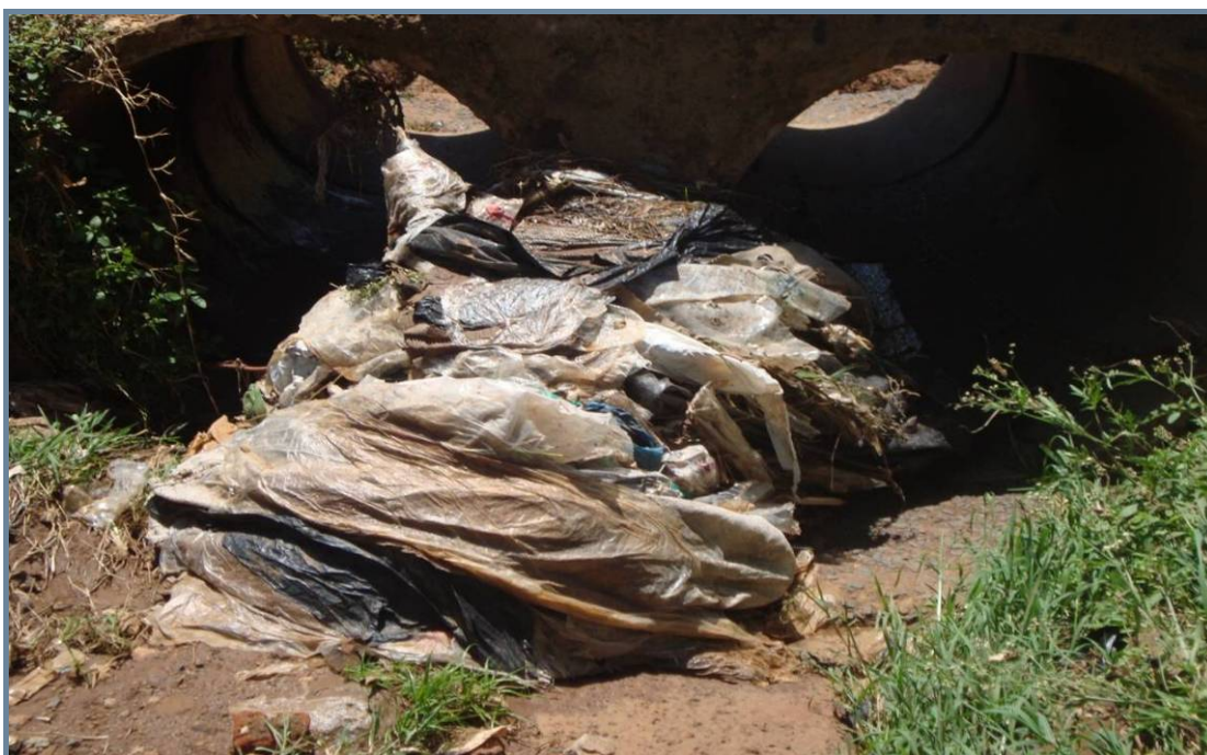
Figure 3-6: A clogged drainage system near the abattoir in Bungoma Municipality
